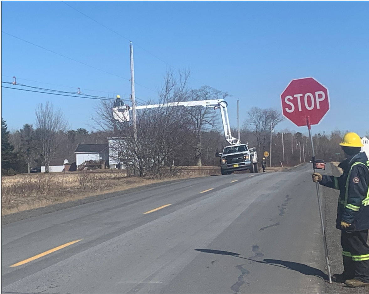
Fibre being installed in Kings County. More than 125 kilometres are now in place.
