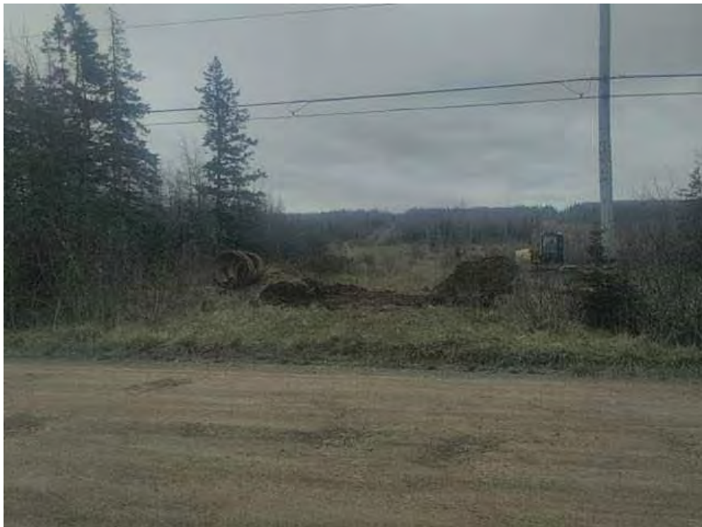
Photo 4. Removal of berm in front of access road to MW1 background location (May 11, 2022).
