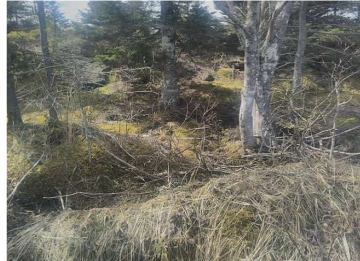
Photo 2. Two of two discharge points to Lake Enon (May, 2022).
